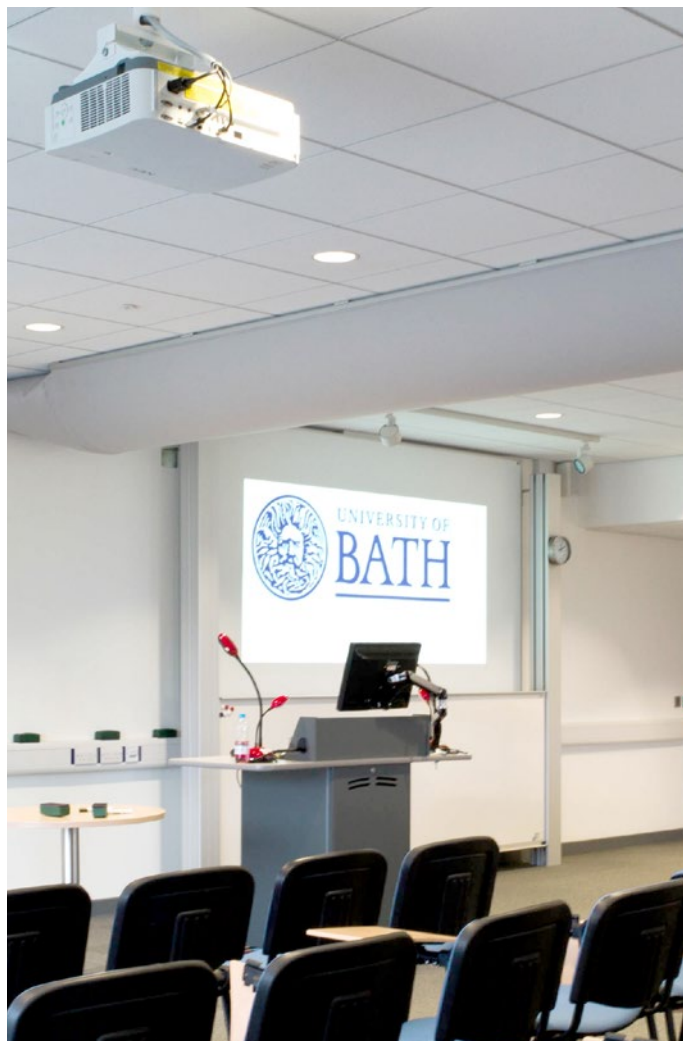
P502HL Laser projector installed across teaching areas at the University of Bath, United Kingdom
